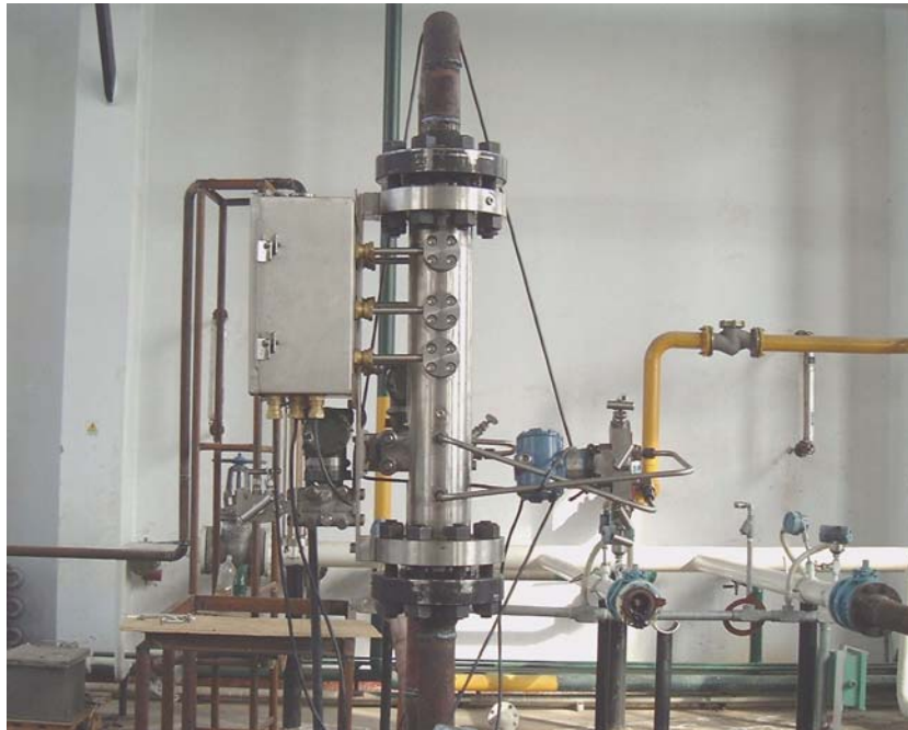
FlowSys MPFM during testing in DOD
